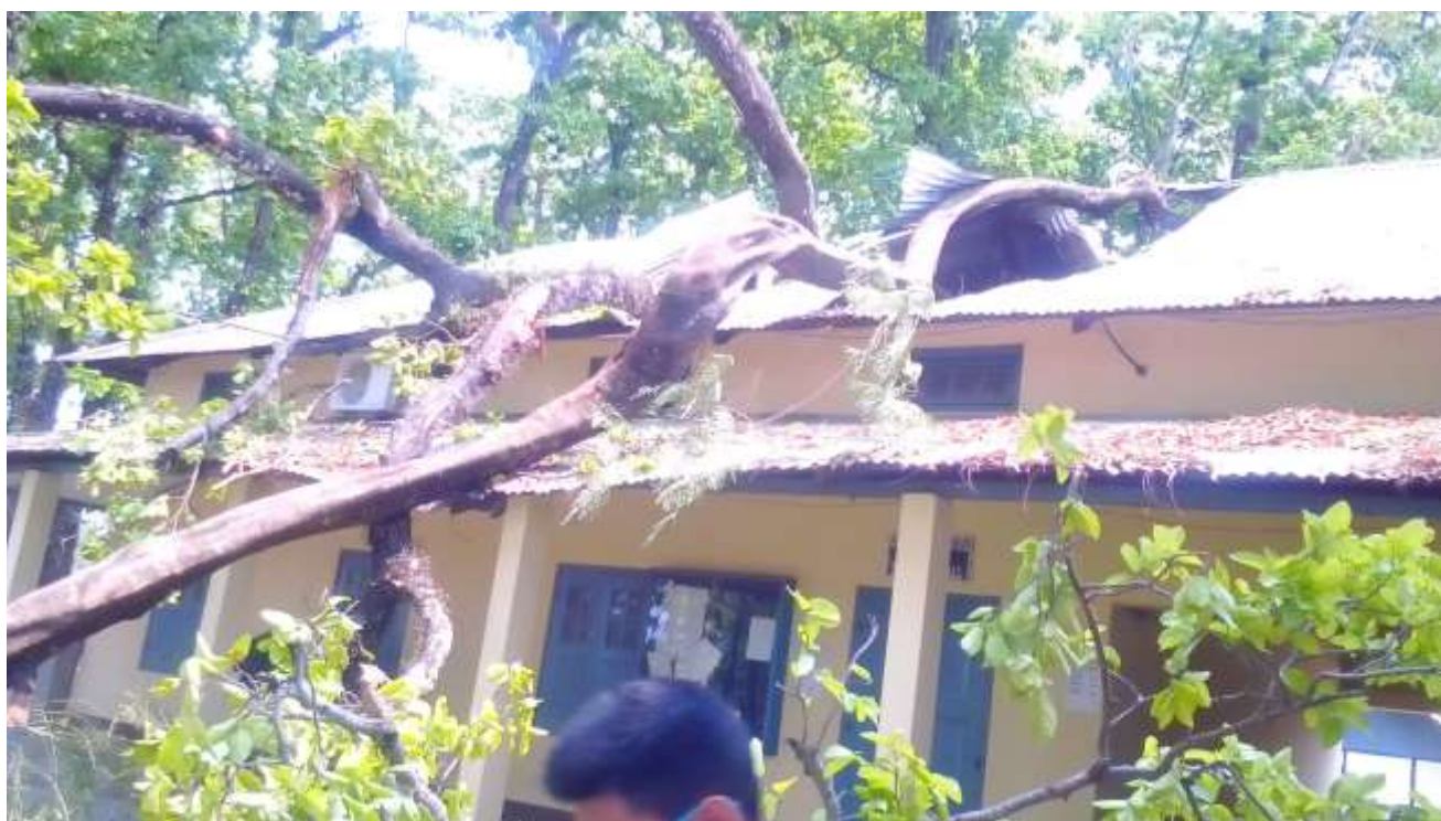
Showing havoc caused due to wind fall Sal Tree
